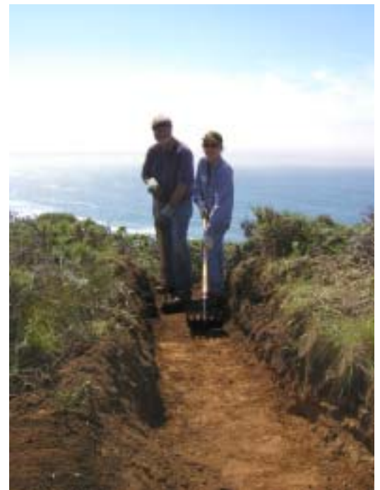
Dave Taylor and Jennie Mollica showing off their new drain. Photo by Hank Magnuski.
