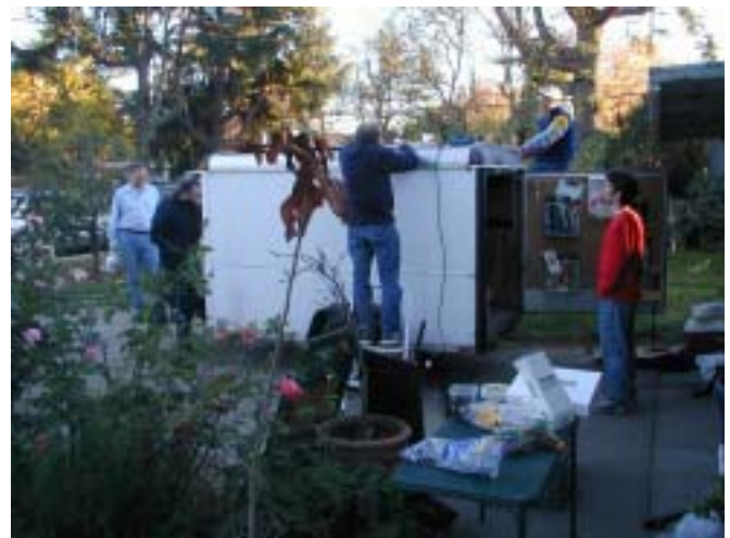
Volunteers reroofing the tool trailer at the November 22, 2003 tool party. Photo by Scott Heeschen.
